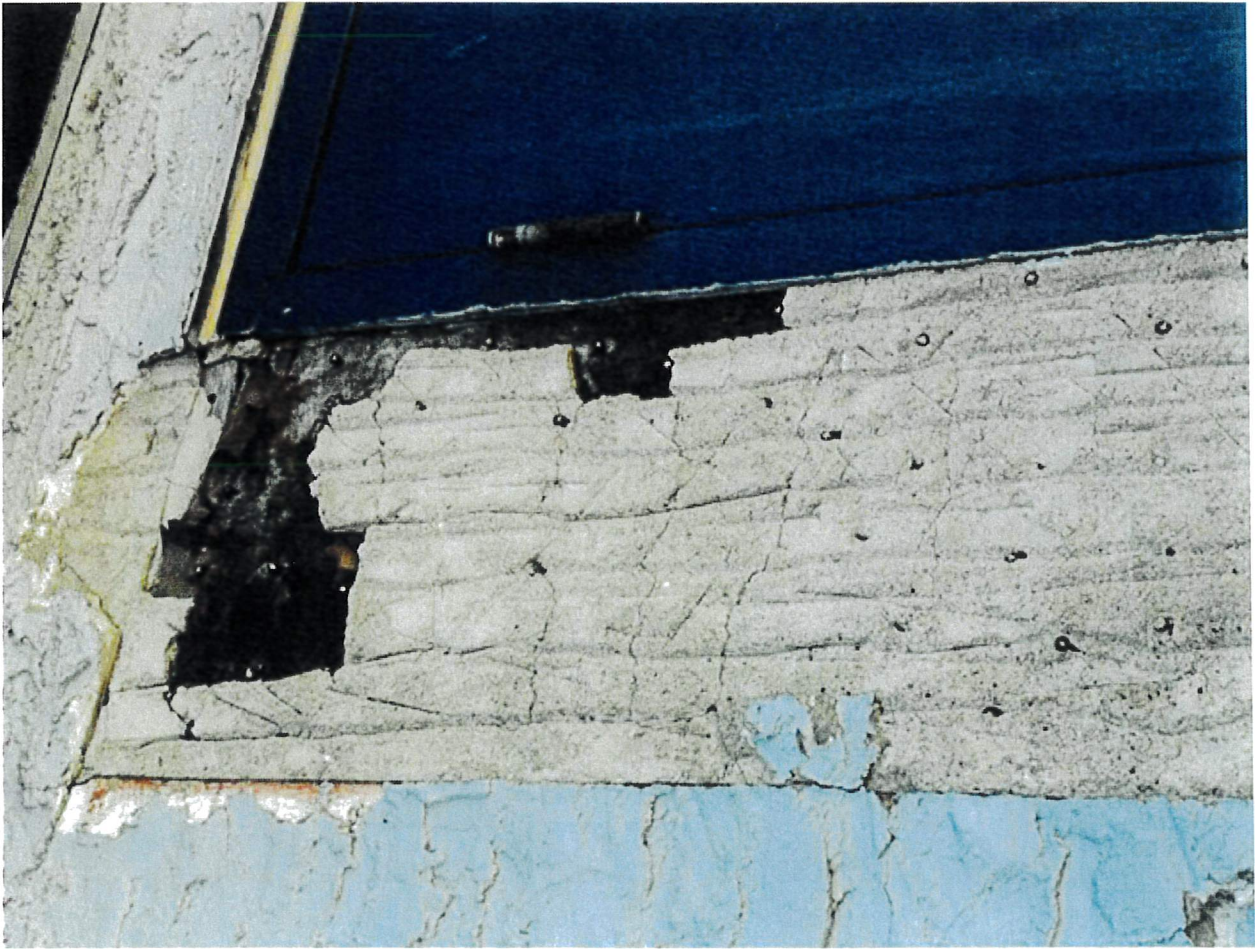
Badly damaged/ deteriorated stucco & plywood behind a wall assembly
