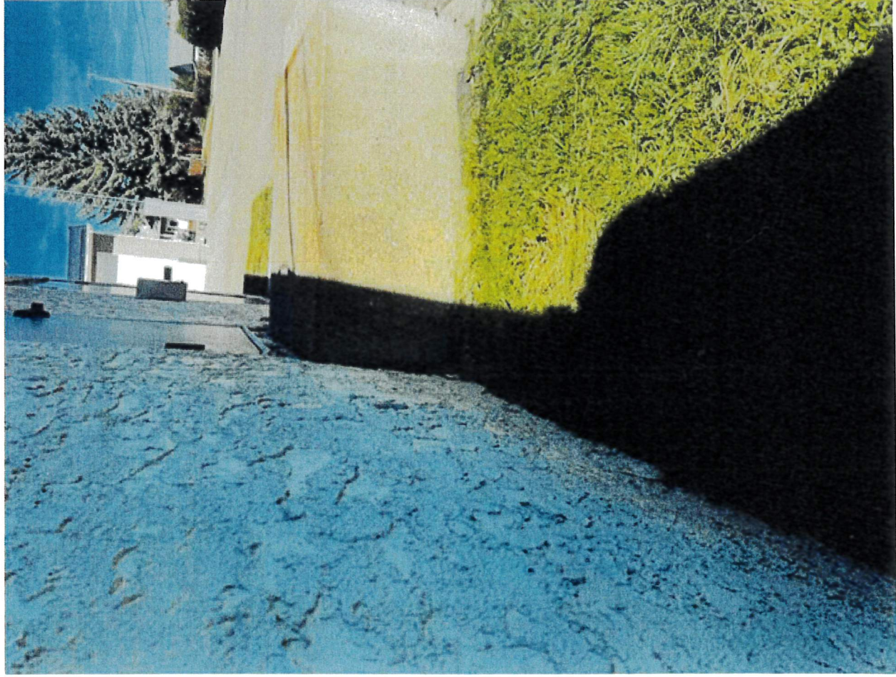
E. Wall PWF wall pushed in ,
