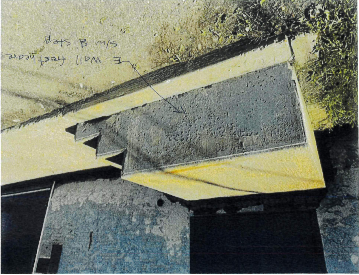
E. Wall damaged stucco & water damage to stucco & behind
