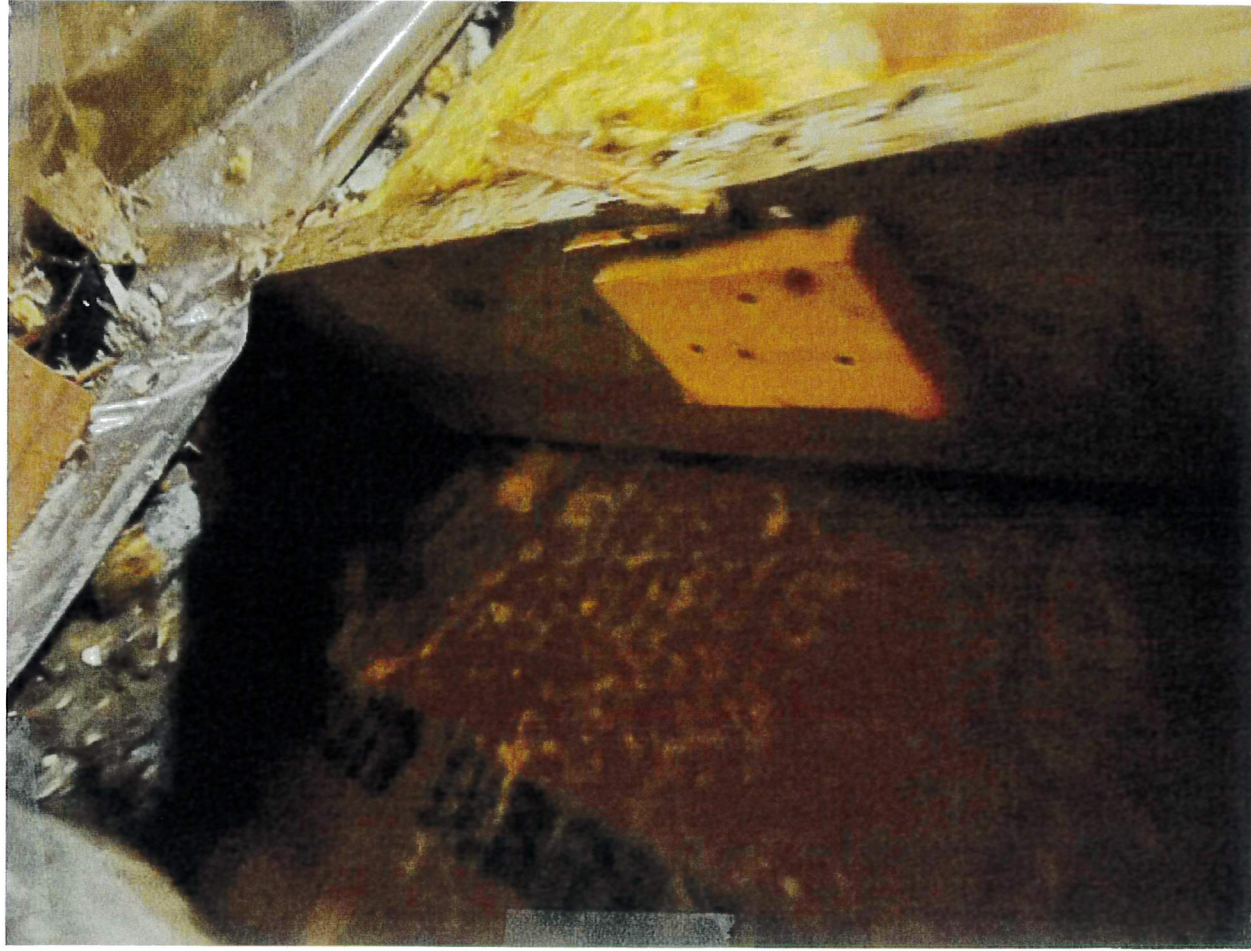
Top Stress cracks on I/F 2x8 PWF Studs
