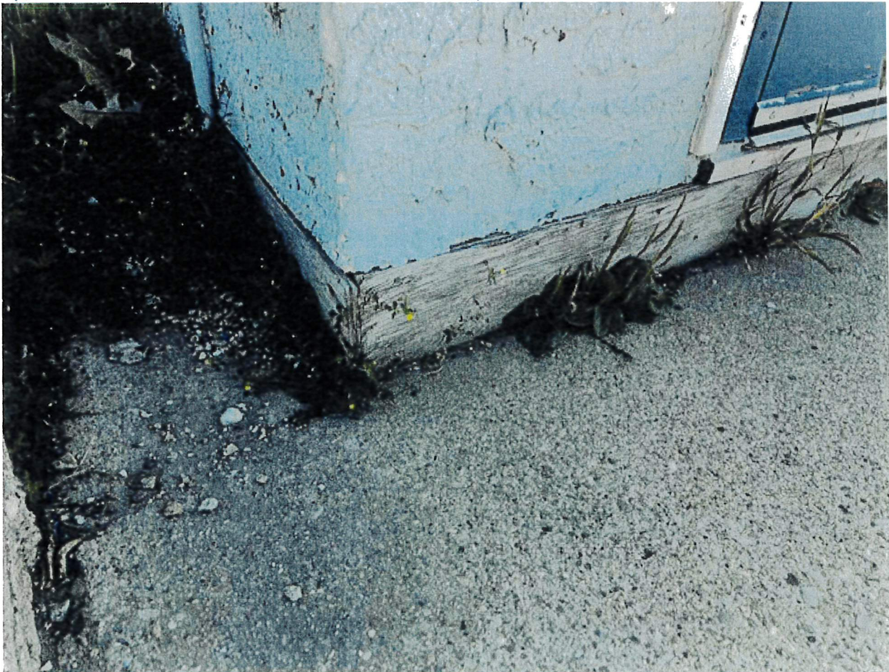
N.W corner Skirt board Shattered & rotten
